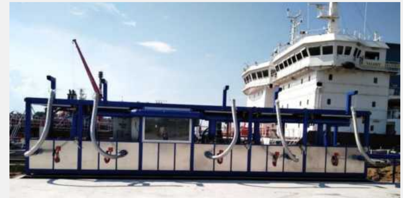
AUTOMATIC TANKER TRUCK UNLOADING POINTS FOR 6 POINT INSTALLATION
